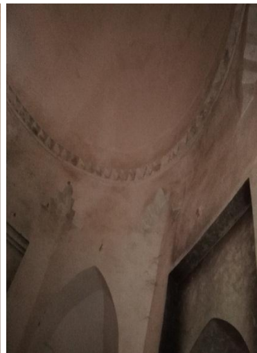
Figure 7: one side internal half hemispherical roof with recessed panels and chevrons are visible.
