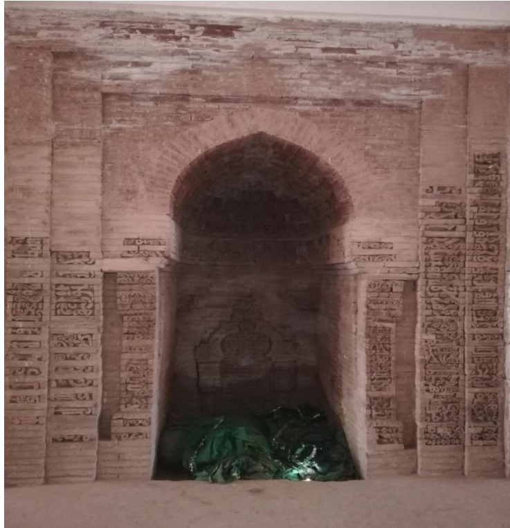
Figure 9: Image of the interior top, middle and bottom of the Mehrib as well as the triple parallel lines of the rubbed bricks flat panels on the facing. These Kufic Script rubbed bricks have been fixed after repairing in which some parts of the flat panels are missed and the top is totally missed.
