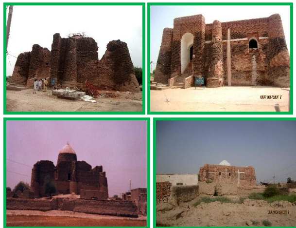
Figure 11: Missing brick masonry on the top of the walls and parapets and repaired
